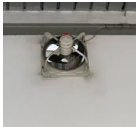
Figure 3. Exhaust Fan inside the B3 TPS room.
